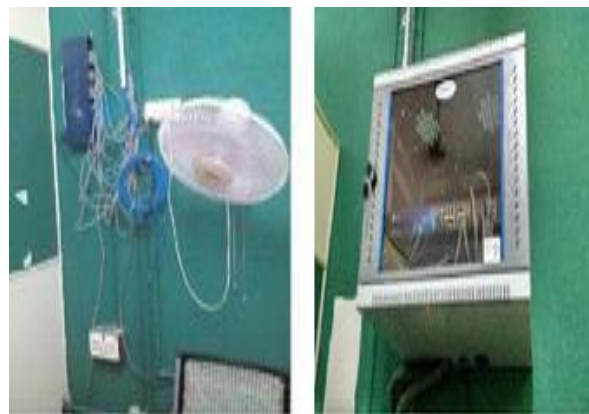
Figure 11 Safety a concern (Before & After)
