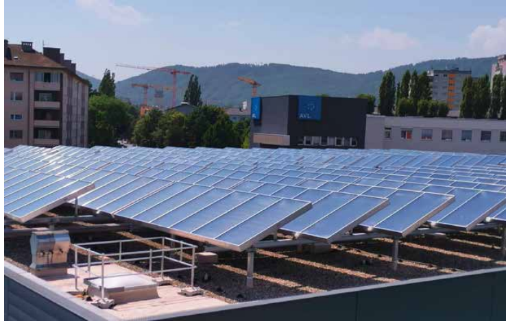
Figure 7. Roof mounted 3 500m 2 of flat plate solar collectors supply heat to drive a 660 kW absorption chiller at the company AVL in Graz, Austria (Weiss and Spork-Dur, 2022)
